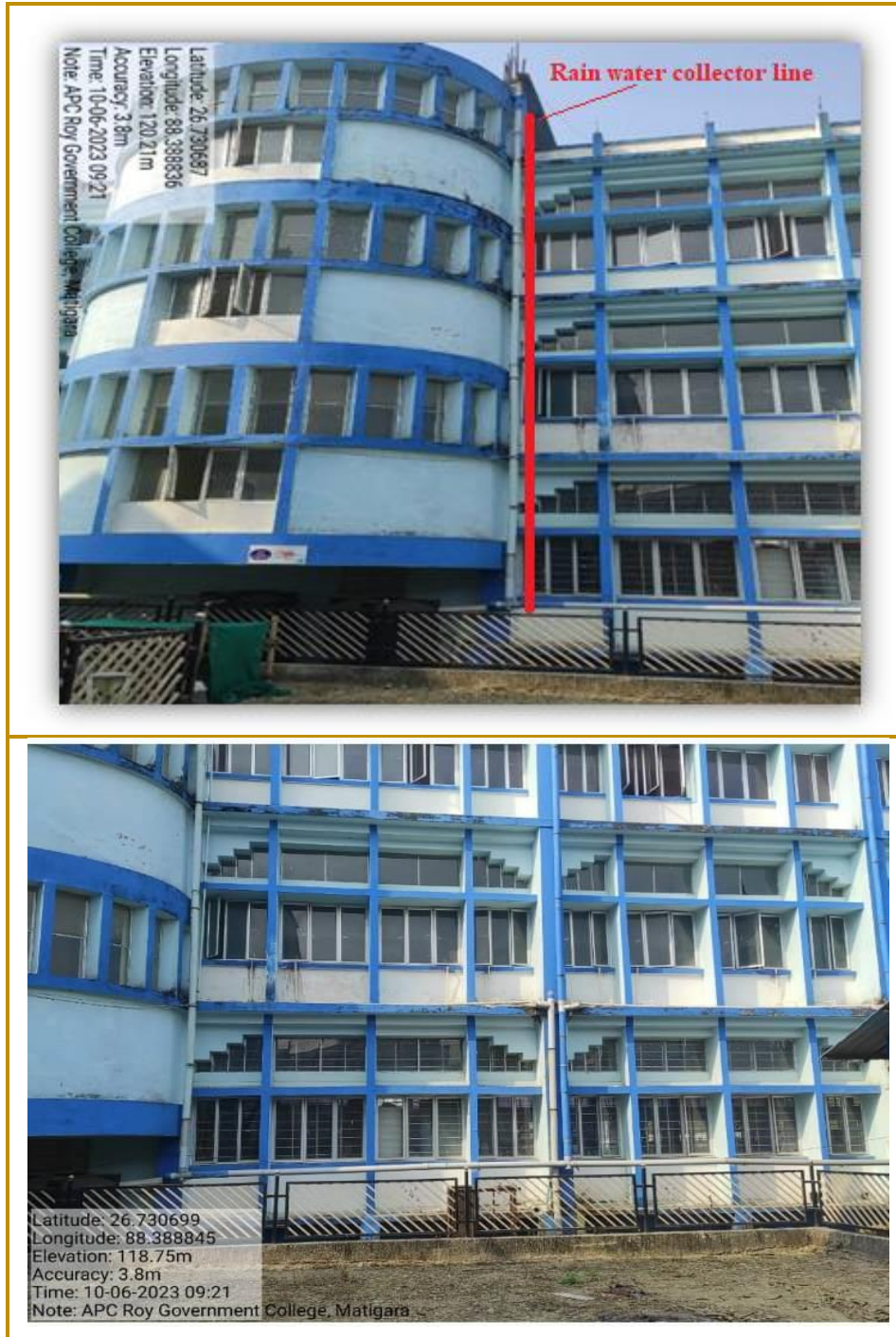
Fig 3: Rain Water collecting lines
